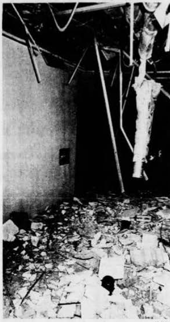
Blown-away ceilings and bent steel beams testify to the power of a bomb that struck a Mobil office in Eastchester seconds after evacuation.
